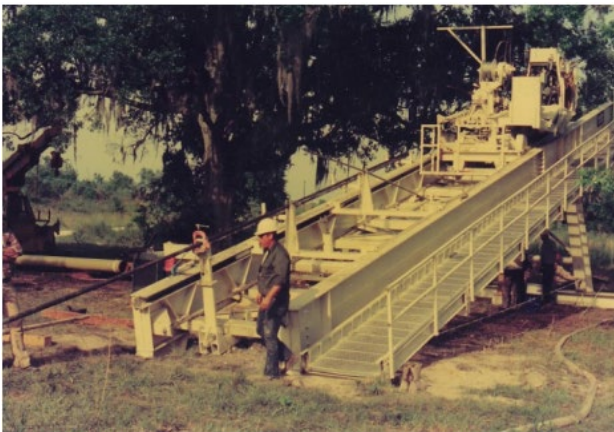
Cherrington's first HDD rig build for a river crossing, shown here working on a series of river crossing projects for Dow Chemical in Louisiana in the early 1970s
